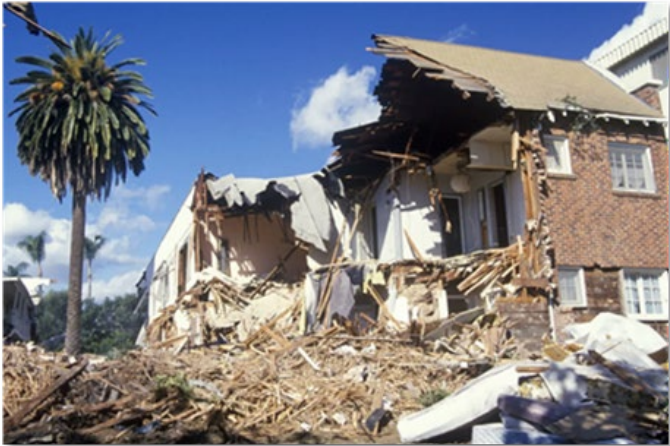
Damage from the 1994 Northridge earthquake
