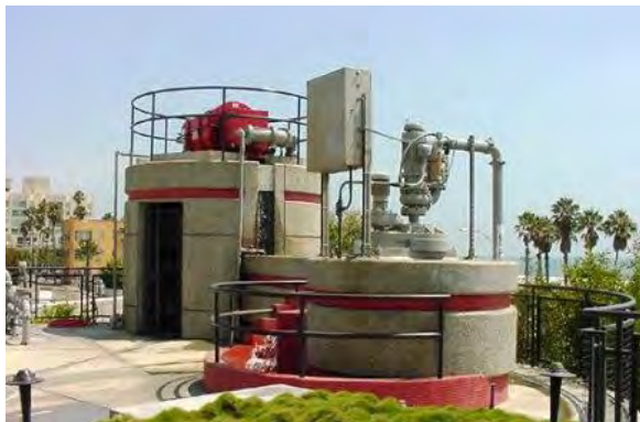
SMURRF Facility. (Source: City of Santa Monica)
