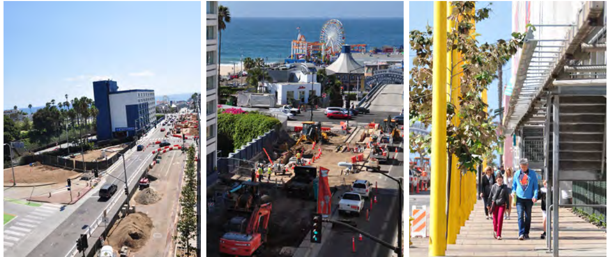
Phasing is an important aspect of project design, particularly for long-range planning documents that span many years and contain a great deal of implementation actions. The Colorado Esplanade, a project, was phased to allow for traffic to continue on Colorado while the street was transformed.
