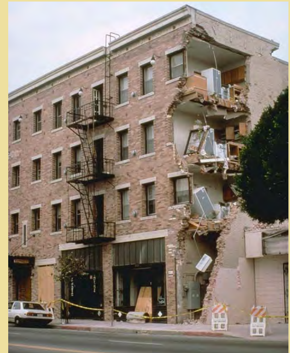
Damage caused by the Northridge earthquake affected many communities around the region.
