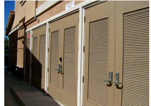
Illustrative image: Mechanical equipment attractively screened at the rear of the building facing Alley.
