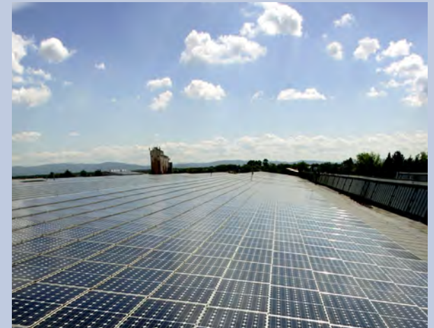
Santa Monica’s ambitious goal to reach “zero net” energy use by 2020 will require strict new construction requirements, as well as an investment in retrofitting existing facilities.
