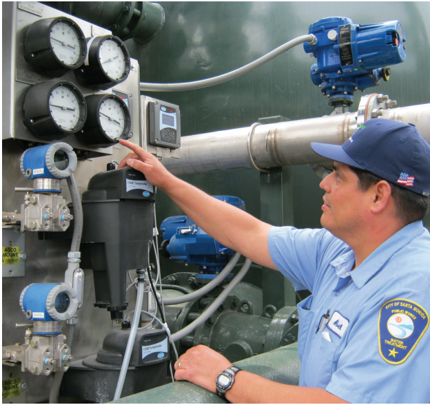
Plant Operator verifying analyzers associated with Iron/Manganese removal.
