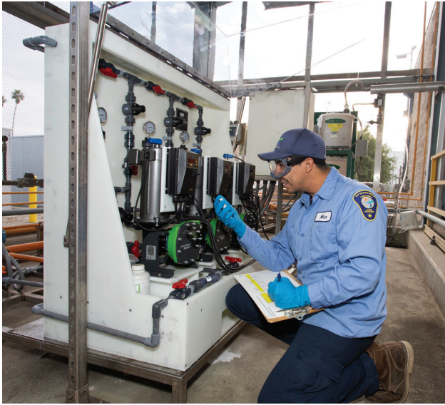
Plant Operator on daily rounds verifying chemical pump dosage.
