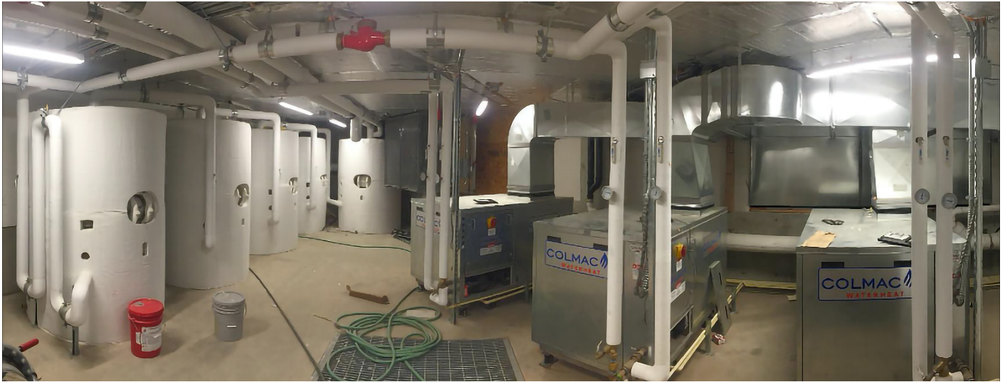
Central HPWH equipment with 2500 gallons storage located in a parking garage in the Batik Apartments, Seattle, WA (Courtesy of Ecotope).
