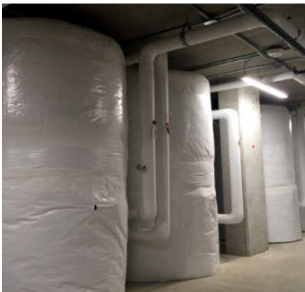
2500 Gallons of Well-Insulated Storage for Cyprus Apartments—230 Market Rate Units (Courtesy of Ecotope).
