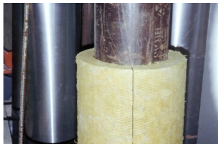
Insulating pipes reduces heat loss in pipes (Courtesy Wikipedia).
