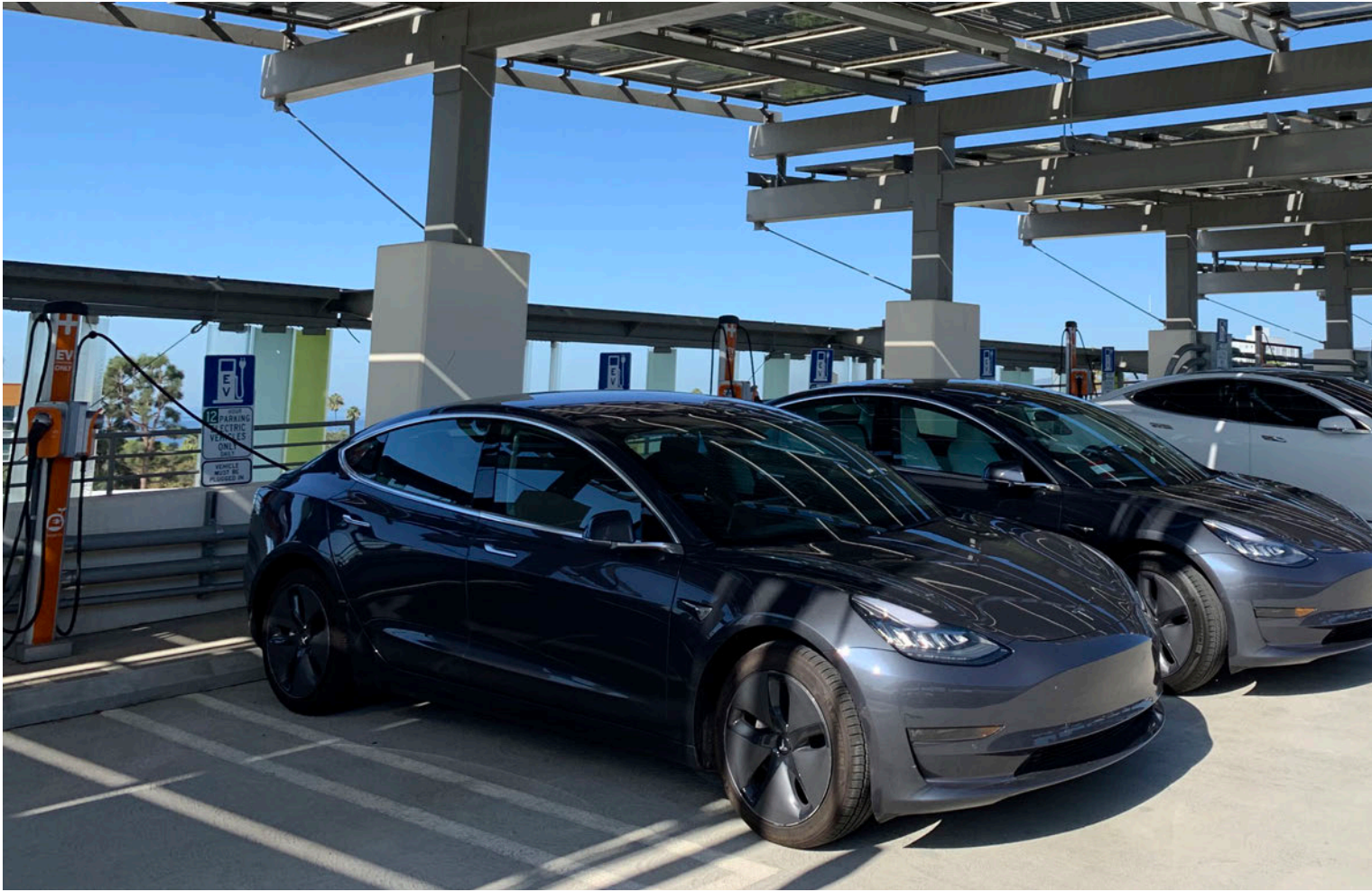
EV charging at the Civic Center Parking Structure in Santa Monica (Courtesy of City of Santa Monica).
