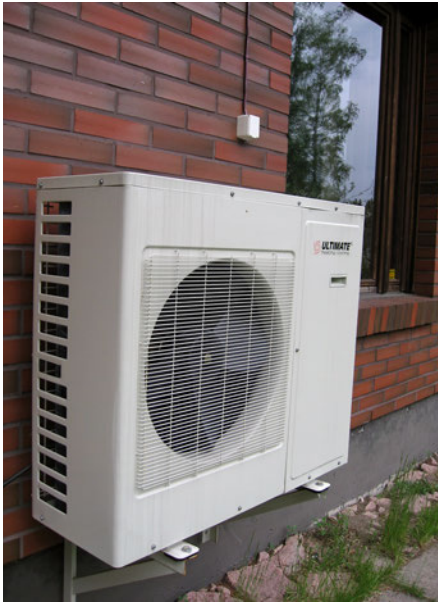
An outdoor unit for a residential heat pump space conditioning system.
