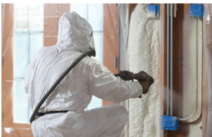
Spray foam insulation can increase comfort by minimizing heat transfer, reducing HVAC loads (Courtesy of Dan Tapia).
