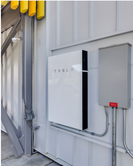
Tesla Power wall battery at the Kienapfel Passive House in Culver City, CA designed by PARAVANT Architects. (Image courtesy of Fraser Almeida)
