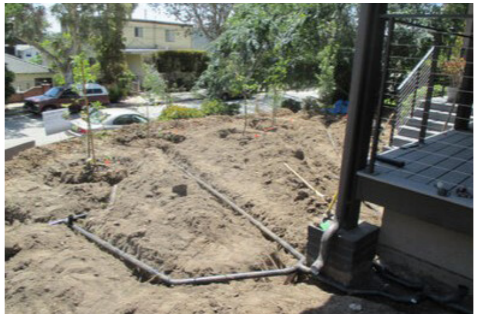
A greywater irrigation system is being installed in Los Angeles, CA. (Courtesy of Greywater Corps)
