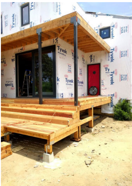
Perlita Passive House in Los Angeles, CA designed by Arcolution LLC. A blower door test is conducted to quantify the amount of air leakage and the effectiveness the air-sealing prior to finishing the house. (Image courtesy of Lawrence Anderson)
