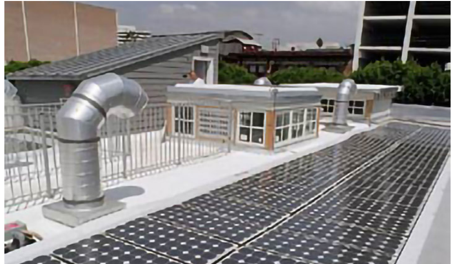
Photovoltaic panels at NRDC Santa Monica Office (Courtesy of Tim Street-Porter).
