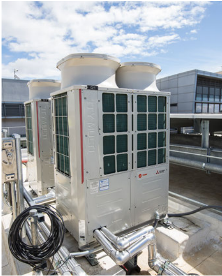
The outdoor unit for a commercial heat pump space conditioning system at the Santa Monica City Hall (Courtesy of City of Santa Monica).
