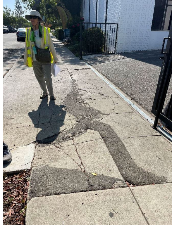
Figure 6. Uneven sidewalks along Pico Blvd.
