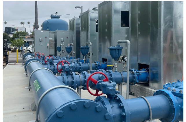
Recently added pump station to meet demand of the City's growing community.
