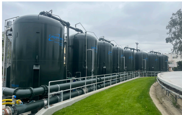
Granular Activated Carbon filters as part of new treatment plant expansion.
