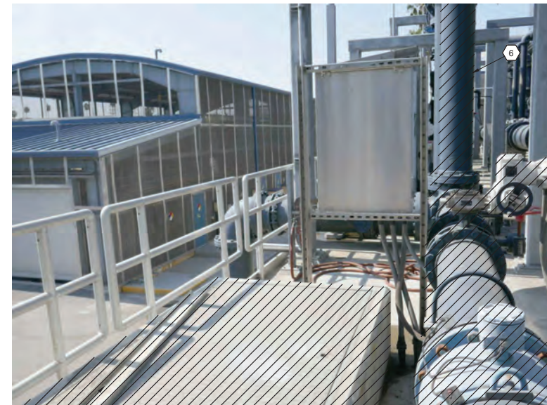
RO BYPASS MODIFICATIONS AND FUTURE RO TRANSFER PUMP LOCATION
