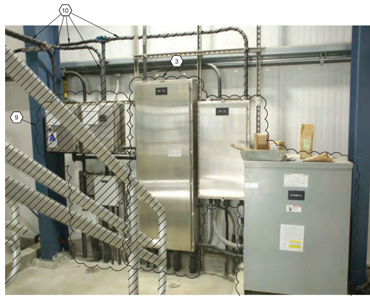
FLOURIDE BUILDING ELECTRICAL PANELS
