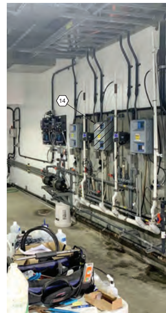
TOTAL CHLORINE ANALYZER AT INLET VAULT (BELOW ELECTRICAL BUILDING)
