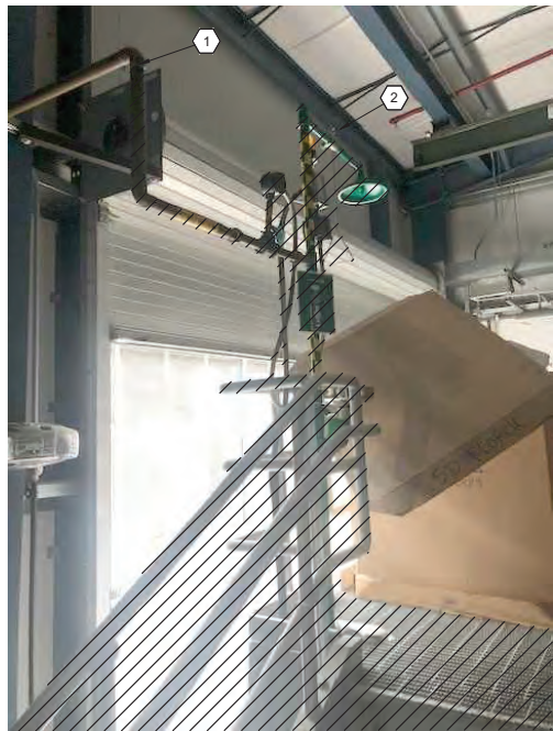
EMERGENCY EYE WASH AND POTABLE WATER PIPING
