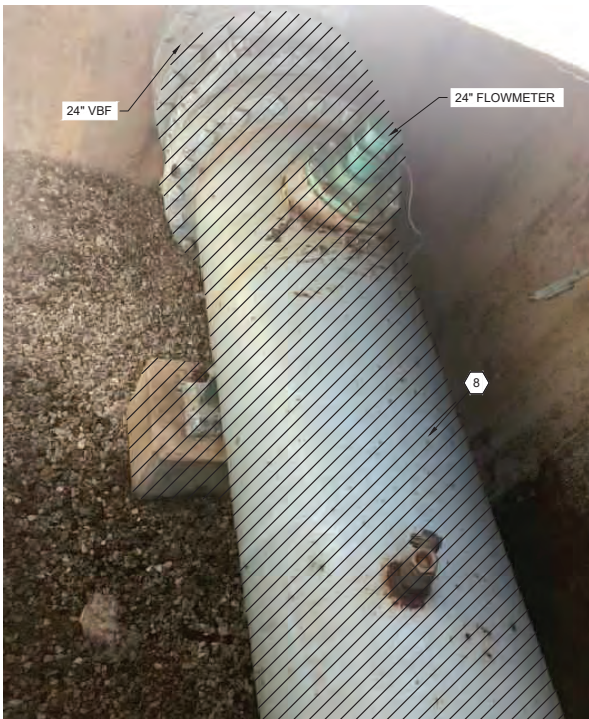
DECARBONATOR EFFLUENT MAGNETIC FLOWMETER
