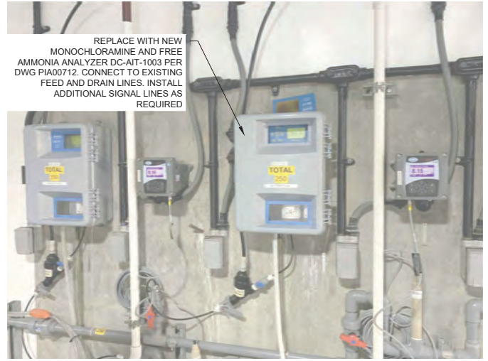
NEW ANALYZER AT INLET VAULT
