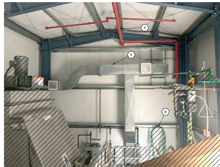
FLOURIDE BUILDING HVAC AND SPRINKLER SYSTEM
