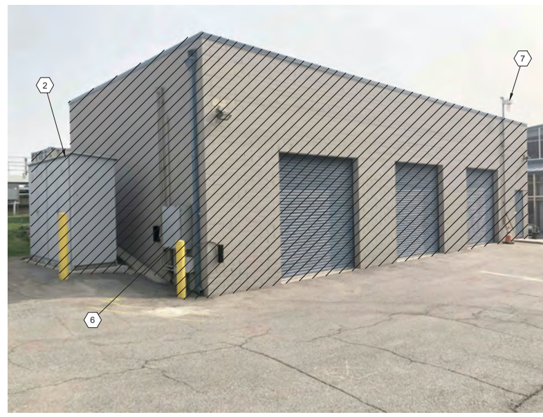
MCC-D AND OUTSIDE OF MAINTENANCE BUILDING
