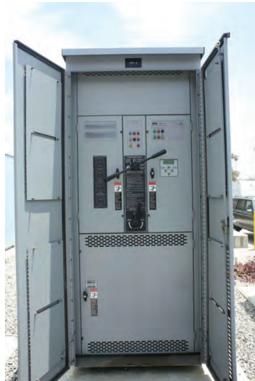
EXISTING TRANSFER SWITCH ATS-A ①
