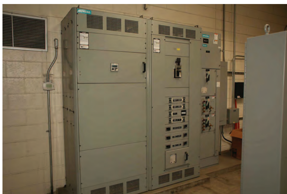
EXISTING SWITCHBOARD SWBD-PF (4)
