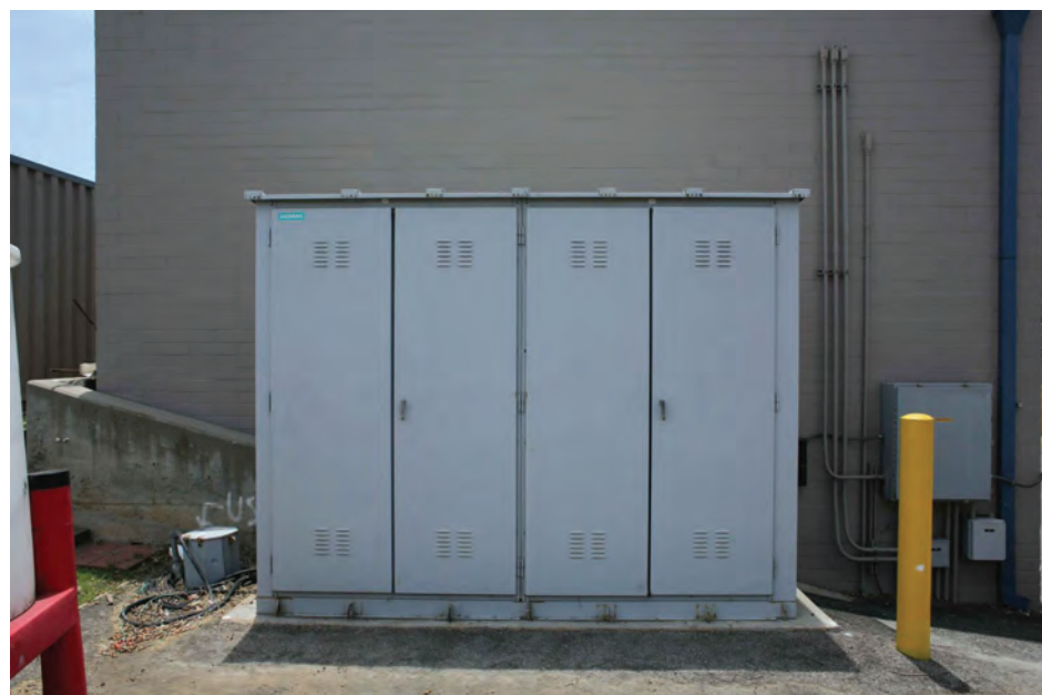
EXISTING MOTOR CONTROL CENTER MCC-D (3)
