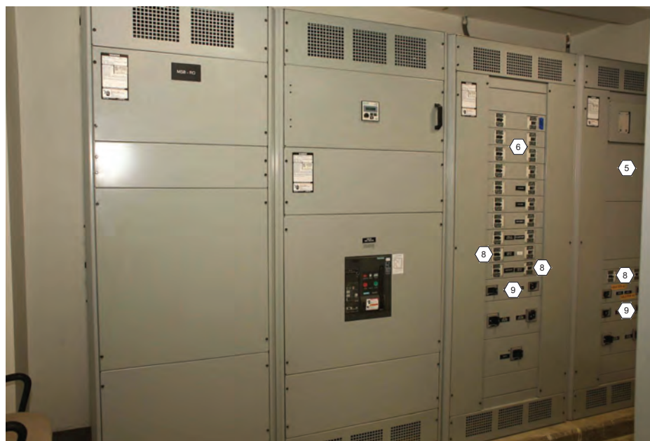
EXISTING SWITCHBOARD MSB-RO (2)
