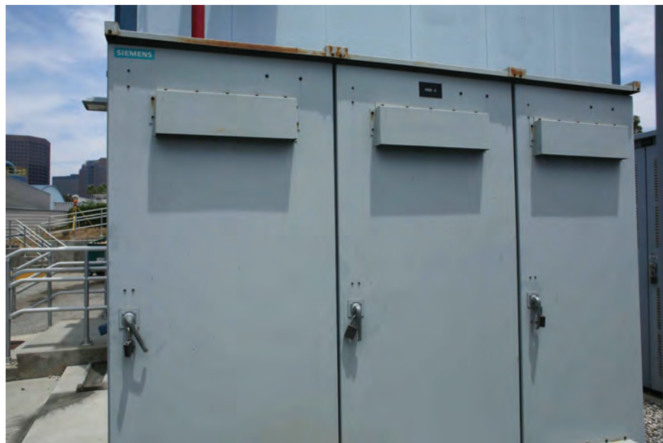
EXISTING SWITCHBOARD MSB-A (1)
