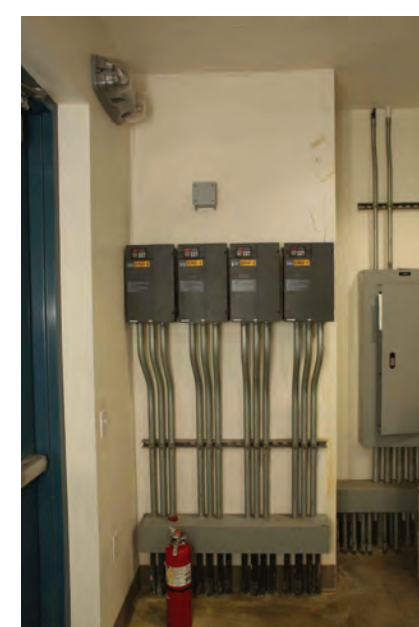
EXISTING ENERGY RECOVERY VFDS (7)
