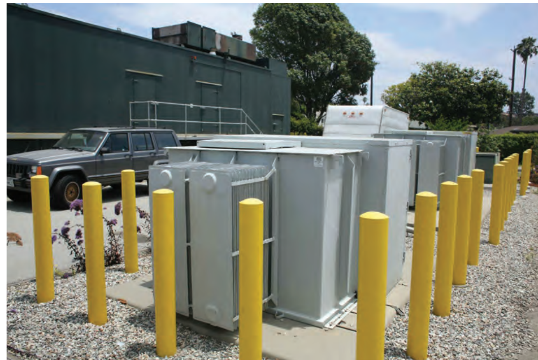
EXISTING LADWP TRANSFORMERS ②
