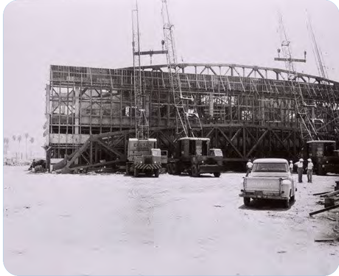
Construction of the Civic Center Auditorium in 1957 Source: Santa Monica Public Library
